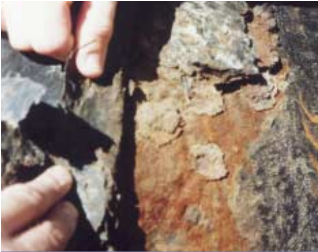
Problem - Failure of original coating system.
